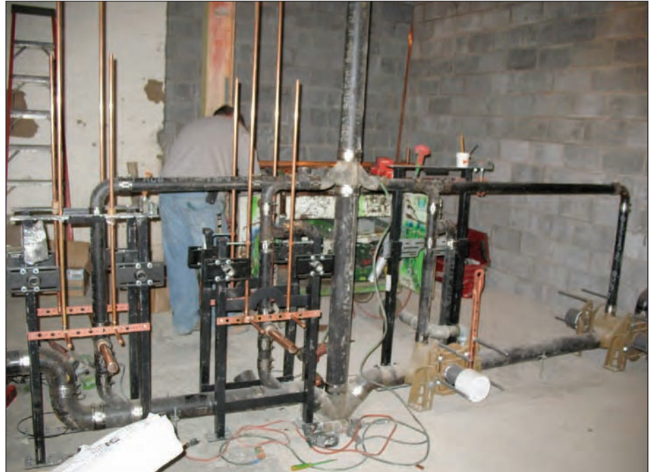
Evans Mechanical uses Jay R. Smith Mfg. Co.'s Labor Saver Fixture and water closet supports for all projects with tight deadlines because they speed up the installation process.
