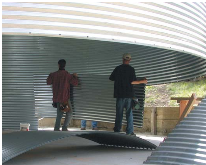
Corrugated tanks are built from the top down. As a row is completed, the tank is raised until the finished tank sits on the concrete slab, is secured, then lined with a NSF-61 potable water membrane.
