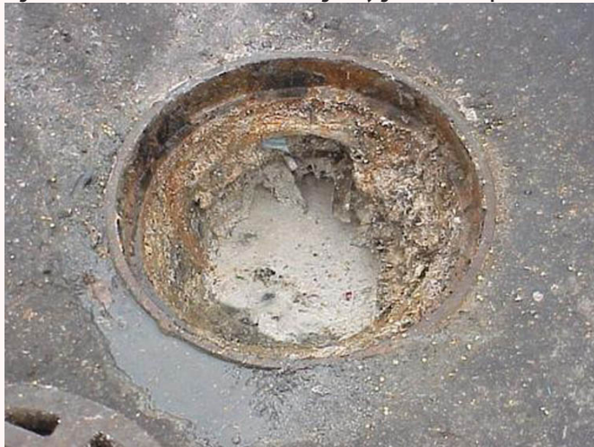
Figure 2 Excessive FOG accumulation in gravity grease interceptor
