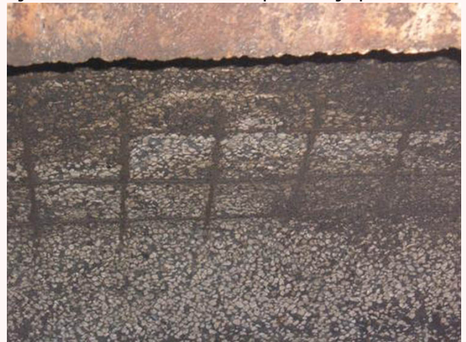
Figure 3 Halo corrosion in concrete interceptor showing exposed rebar
