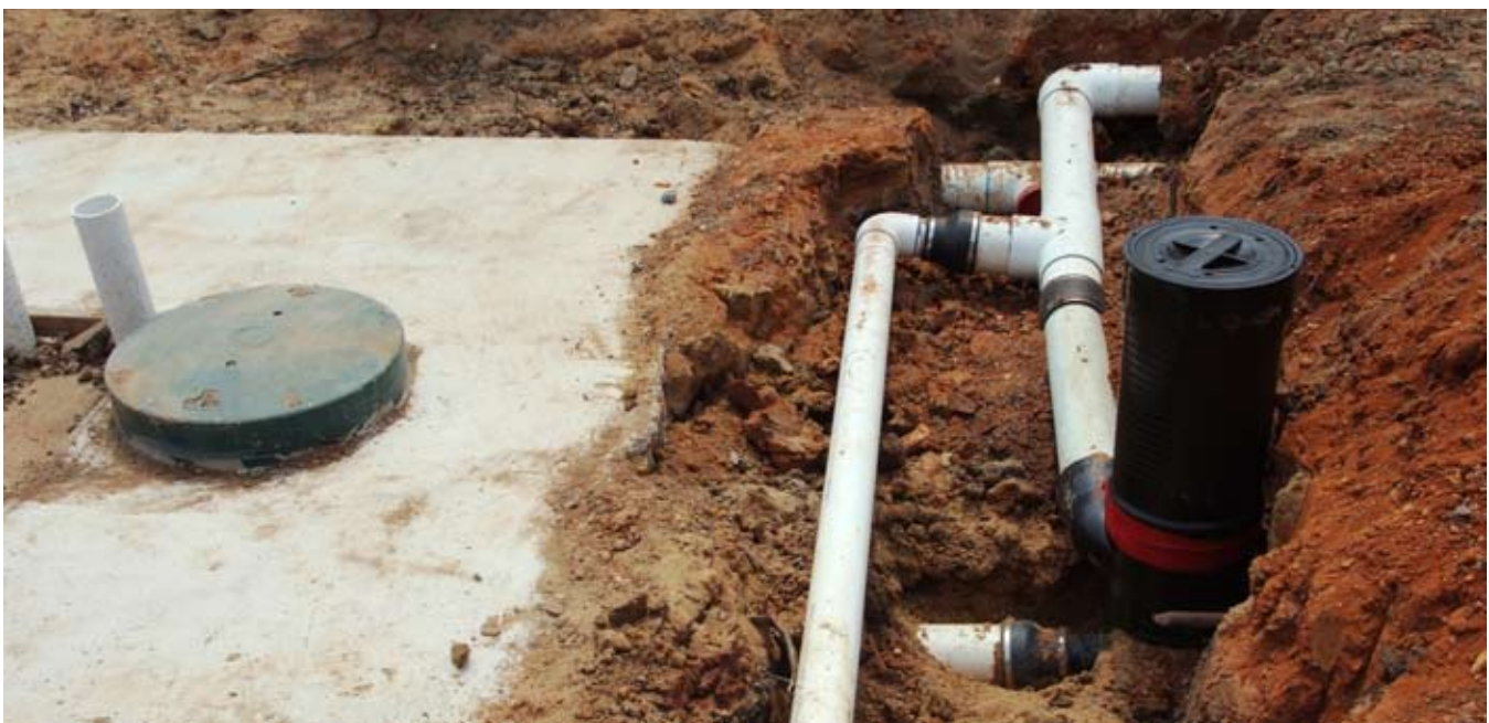
Gerachis' Backyard: Piping from the home to the vortex fine filter, then to the concrete storage tank.
