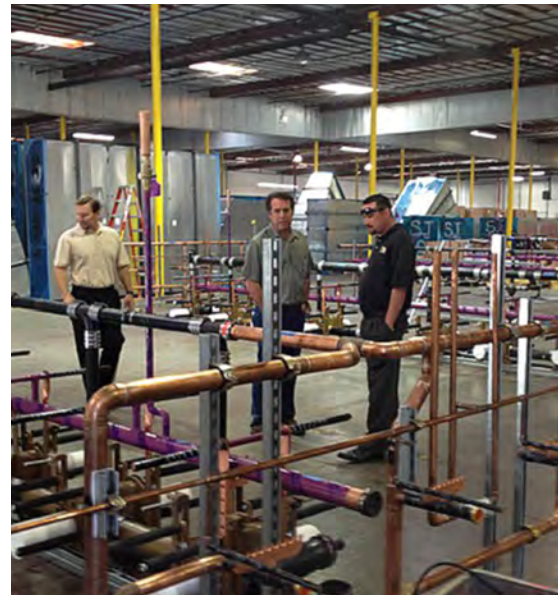
F. W. Spencer & Son relied on prefabrication to ensure smooth, speedy installation of plumbing fixtures to meet the accelerated schedule for the new Levi's Stadium. Jay R. Smith Mfg. Co. Quarterback Water Closet Supports were designed with prefabrication in mind.
