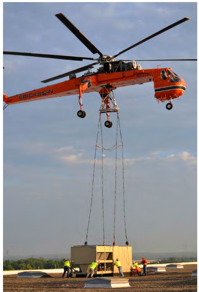
The Erickson Aircrane helicopter placed six air handling units and a condenser on a plant roof in less than one hour, minimizing installation and labor costs for Thomas J. Dyer.
