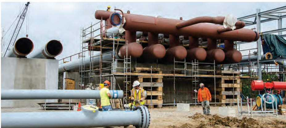
To create precision welds on a tight schedule for a cryogenic natural gas processing and compressor station in the Marcellus and Utica Shales, Sauer Group partnered with Tri Tool Field Services, which developed weld procedures and deployed workers using Tri Tool portable machine tools and AdaptARC multiprocess welding systems.
