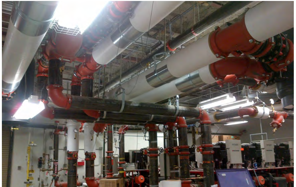
EMC partnered with Victaulic's CPS for BIM, creating isometric drawings that solved unique challenges. For example, laying out piping in 3D allowed EMC to overcome space constraints and include more piping in the mechanical room at Fort Leavenworth.
