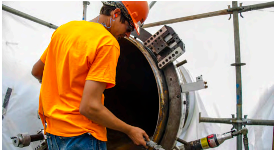
A field machinist makes preparations to ensure a reliable weld on the pipes for a natural gas processing and compressor station. Tri Tool’s attention to quality and safety enabled Sauer Group to perform excellent welds at a rapid pace, meeting the project’s schedule constraints.
