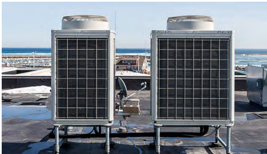
The small footprint and lightweight modularity of Mitsubishi Electric's R-2 Series outdoor units allowed for rooftop installation at the new Franklin Energy headquarters, helping to transform an historic building into a model of energy efficiency.
