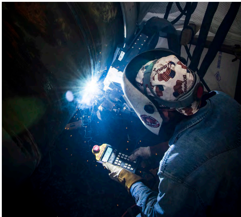
Bottom: Using Tri Tool's AdaptARC system increased Sauer Group's productivity 300 percent over traditional stick welding, saving the contractor two to three shifts of welding time.
