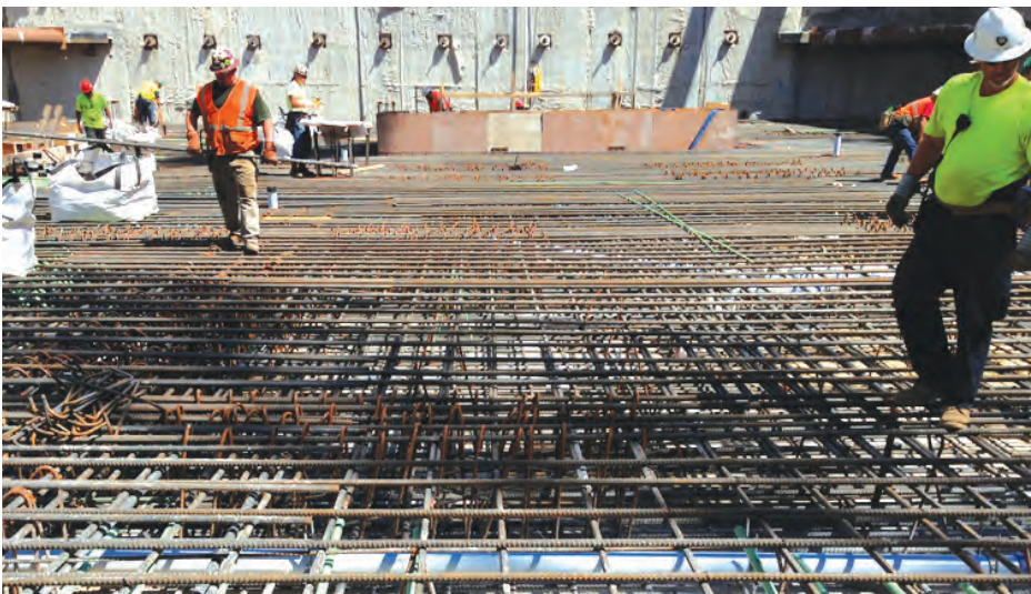
To accommodate any building settling, C.J. Erickson encased all the piping within the concrete slab of the base. They used 3D modeling to set up a grid with all the field layout points. Then all the piping was laid and suspended, and the concrete slab was poured over the piping.
