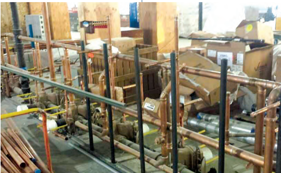
C.J. Erickson used acid-resistant pipes from Jay R. Smith Mfg. Co. throughout a new scientific research center to ensure that all researchers, regardless of the work they were doing, would have the appropriate plumbing in their lab space.
